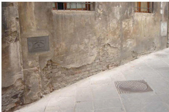
Photograph 2: Spalling of sacrificial layer in Siena, Italy
