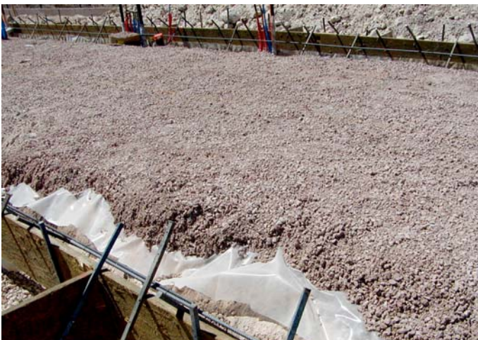
Photograph 2: Slab-on-Grade Done Wrong
