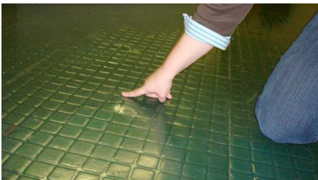
Photograph 9: Failing Vinyl Composition Flooring
