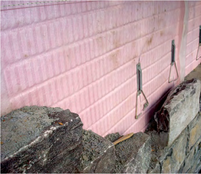
Photograph 6: Above Grade Draining Insulation— Extruded Polystyrene (XPS). The stone veneer is installed with no gap against the exterior face of the draining XPS. The grooves are covered with a filter fabric to keep mortar out of the grooves.
