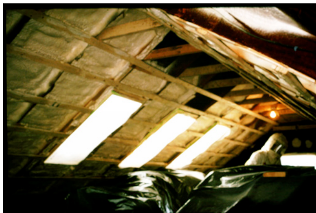
Photograph 4: Spray Polyurethane Foam Attic Retrofit – This is a phenomenal approach to air sealing a building and saving energy. Because of its very effectiveness a ventilation system needs to be installed in conjunction with the work and source control needs to be employed. Don't be stupid. You can't have civilians in the house when the SPF is being applied and the workspace needs to be ventilated during application and after application as you would ("should") when repainting a room or installing new carpet or gluing down flooring or any VOC intensive work. You can't leave existing ceiling insulation in place because of the junk that is in it that has accumulated over countless decades. You have to clean these old insulated surfaces to get rid of the bad stuff. Get rid of standard combustion appliances - install sealed combustion appliances. And for Pete's sake fix the wet basement before you do the work in the attic.
