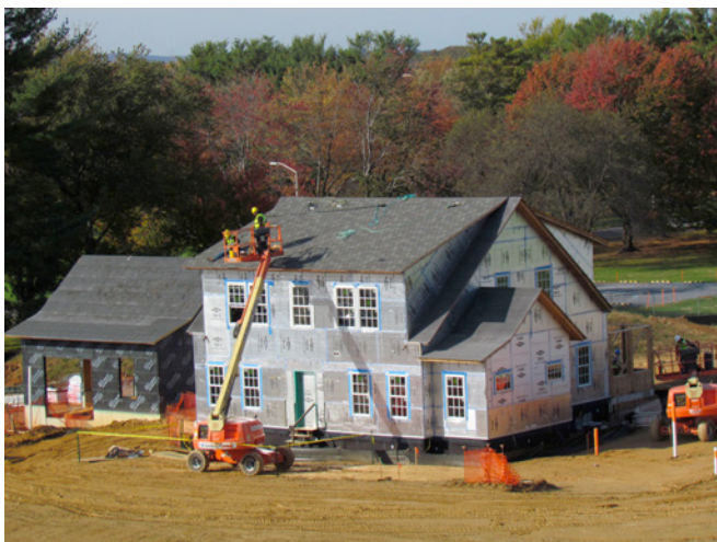
Photograph 2: More Ultra Tight House – Continuous exterior insulation installed over fully adhered exterior air control layer to control condensation at the exterior air control layer – structural sheathing interface. Note that the garage is not attached to the house. Good idea, but typically not possible.
