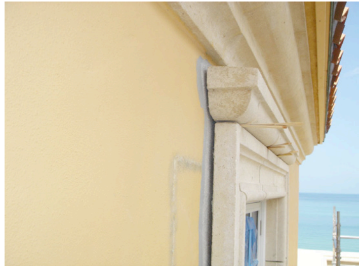
Photograph 4: Precast Trim (above) —It is absolutely critical to drain the back surfaces of these trim elements to prevent perched water and resulting hydrostatic pressure. There are countless sad stories of trim catching water at window to wall interfaces leading to wind driven rain driving forces in the absence of wind.
